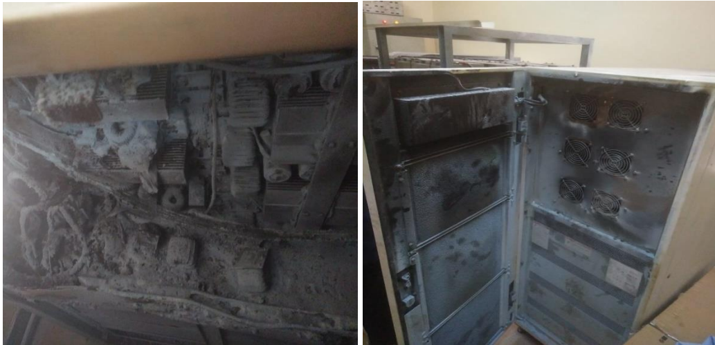
Figure 4. Condition of the UPS in the surgical building of regional general hospital Dr. Saiful Anwar Malang after the fire occurred
