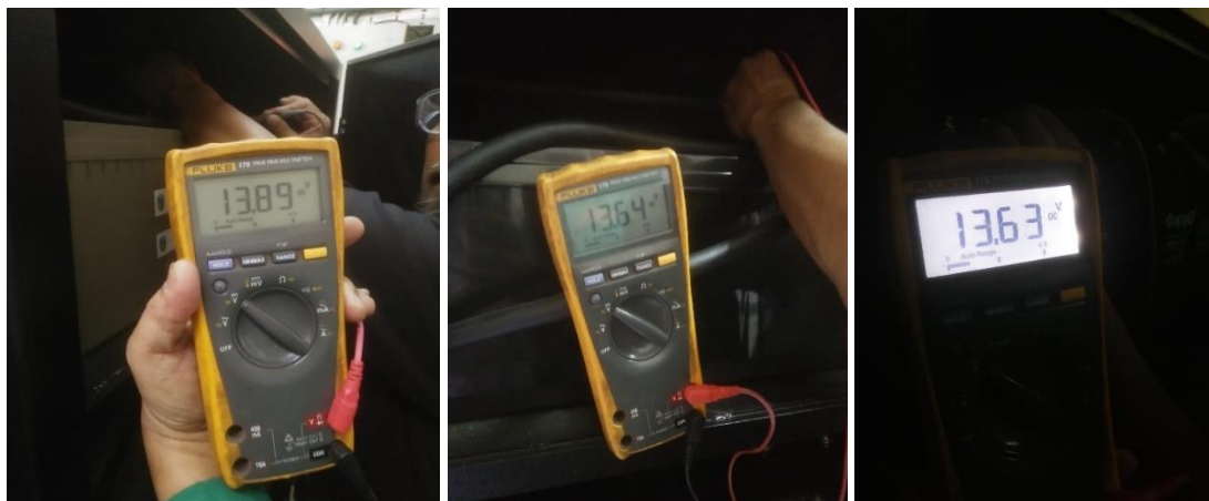
Figure 3. Measure the condition of the UPS on the part of the battery that is overcharged
