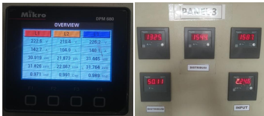
Figure 6. Monitoring voltage and current parameters that indicate unbalanced load
