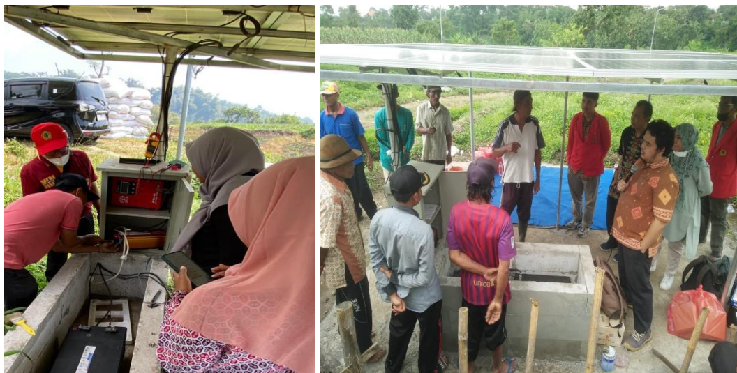
Figure 3. Provision of Solar Power Plant Maintenance Materials
