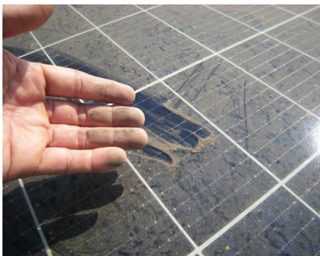
Figure 4. Dusty condition of Photovoltaics
